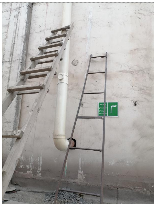
热端喷涂废气排气筒
